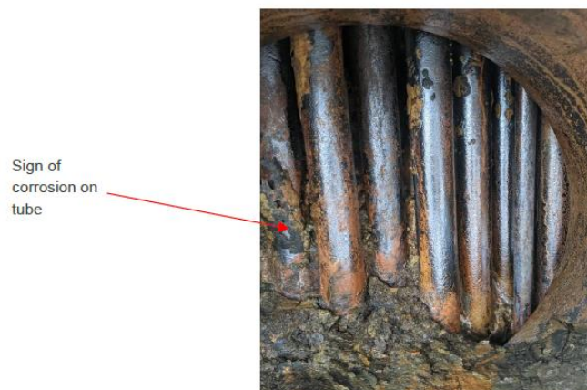
Figure 8. Signs of corrosion on inter-stage tubes.
