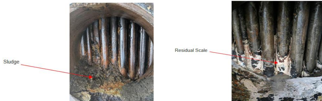
Figure 7. Left: Sludge, Right: Residual scale post acid wash.
