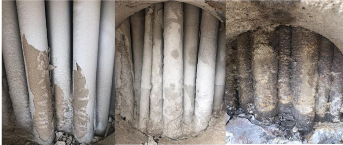
Figure 3. Shell side condition of inter-stage coolers due to poor cooling water quality and delayed maintenance.
