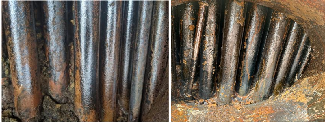
Figure 5. Shell side condition post acid wash.
